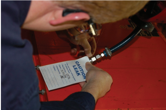
Figure 10-11 Detect and identify leaks.
